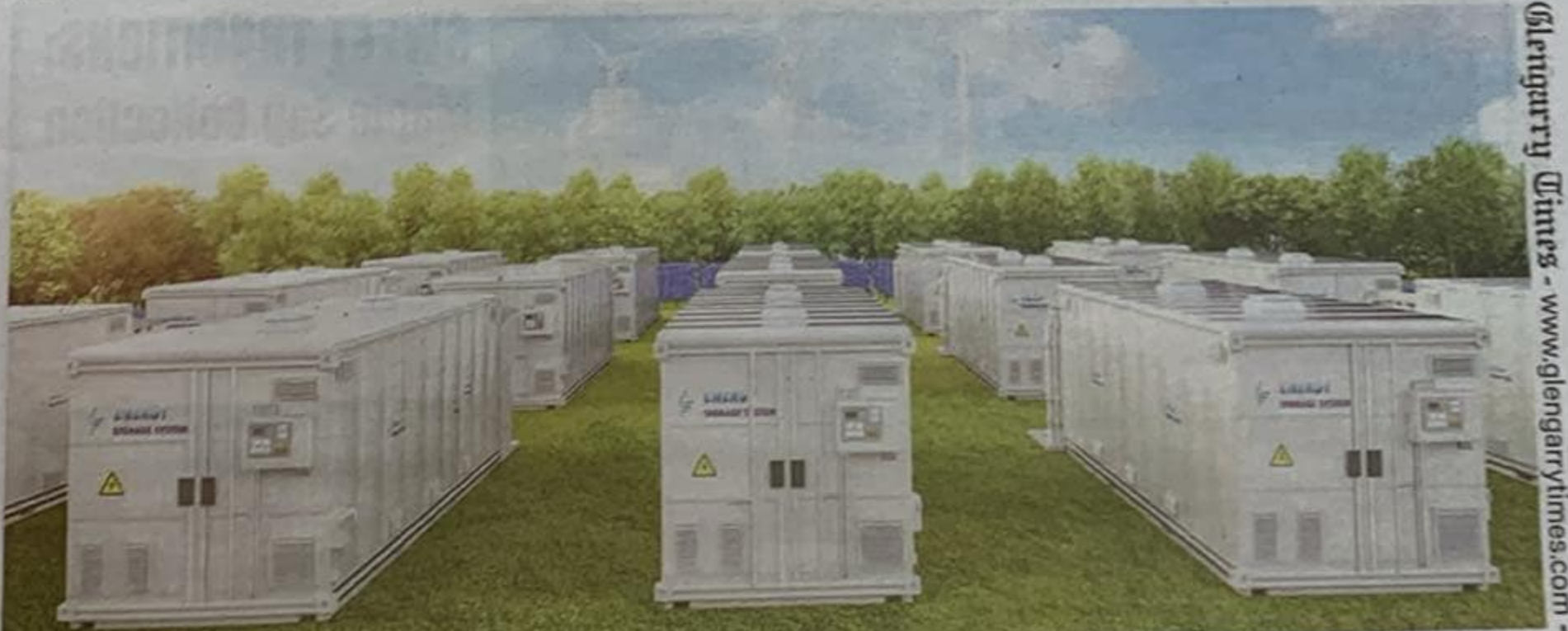
Please note that this image is of a different BESS facilities and may not exactly represent the final design of the Dunvegan project.
